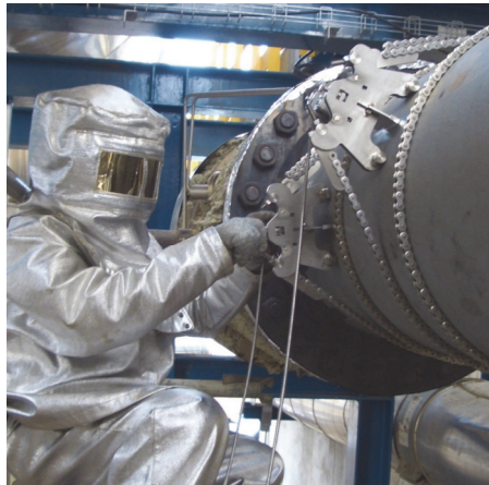
"Hot commissioning" in the truest sense of the word – at pipe wall temperatures of 400 °C.
